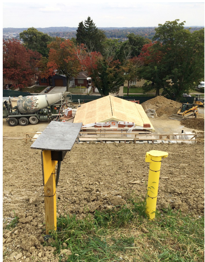
In-place inclinometer installed at site with wireless datalogger
